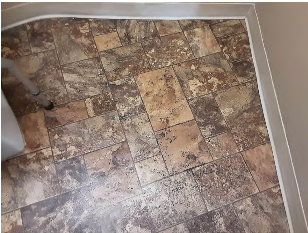
S0034A (Confirmed Asbestos), Floor, Vinyl Sheet Flooring, Tenant Room (Location #: 71)
