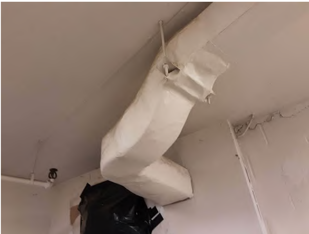
S0056C (None), Duct, Thermal Insulation, Maintenance Shop (Location #: 166)
