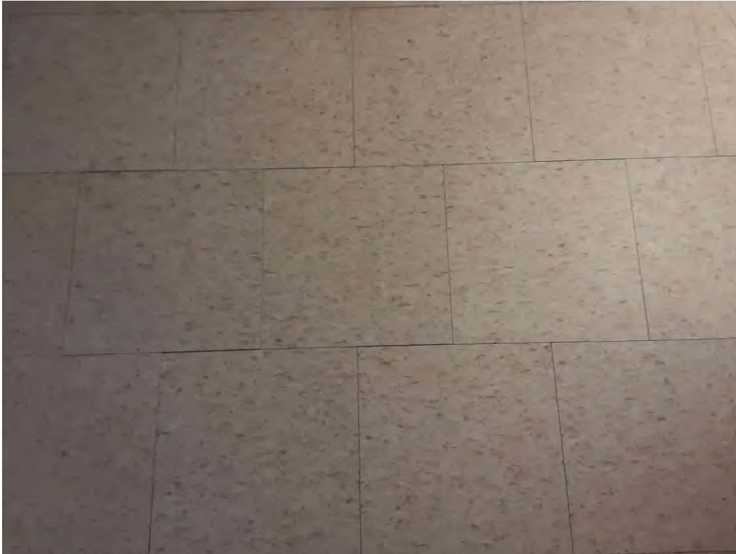
S0023A (None), Floor, All, Vinyl Floor Tile and Mastic, Tenant Room (Location #: 16)
