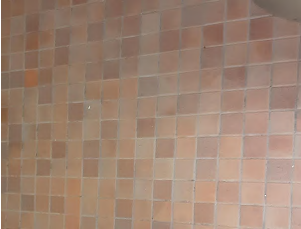
S0080A (Confirmed Asbestos), Floor, Mortar, under 1" x 1" red brick ceramic tile, Women's Washroom (Location #: 114)
