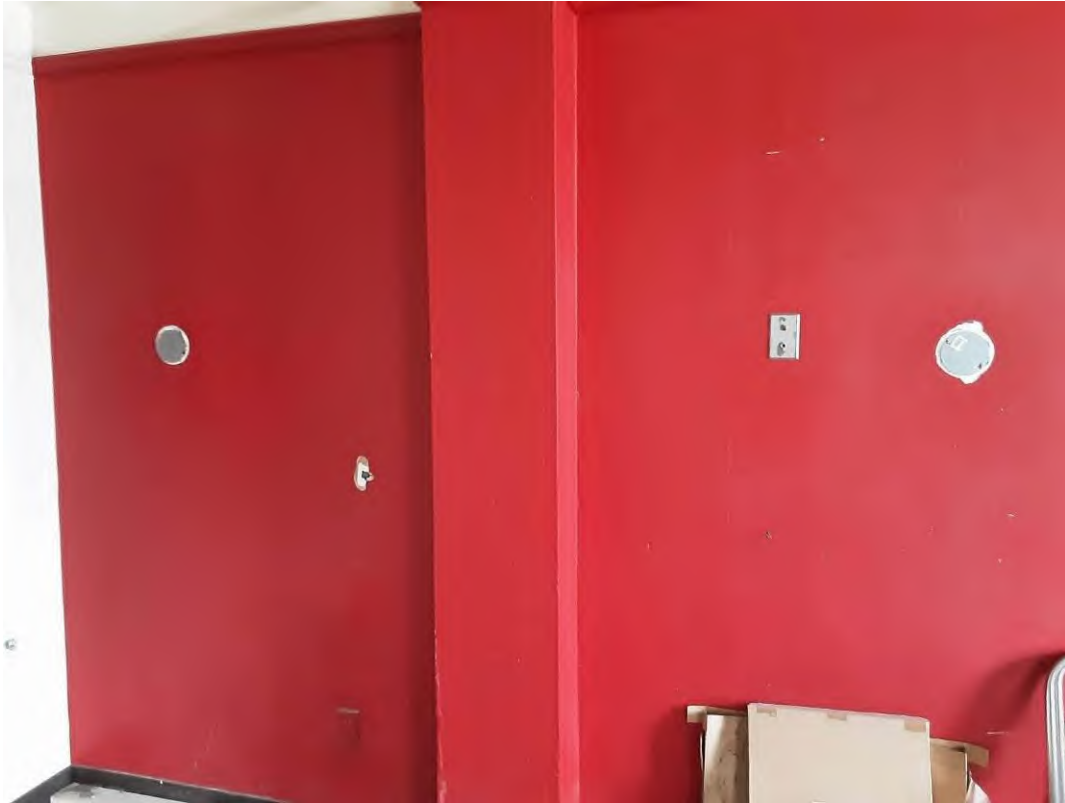
Drywall and joint compound, Red, L0017(Lead (High)), Old House - Ground Floor (Location #: 177)
