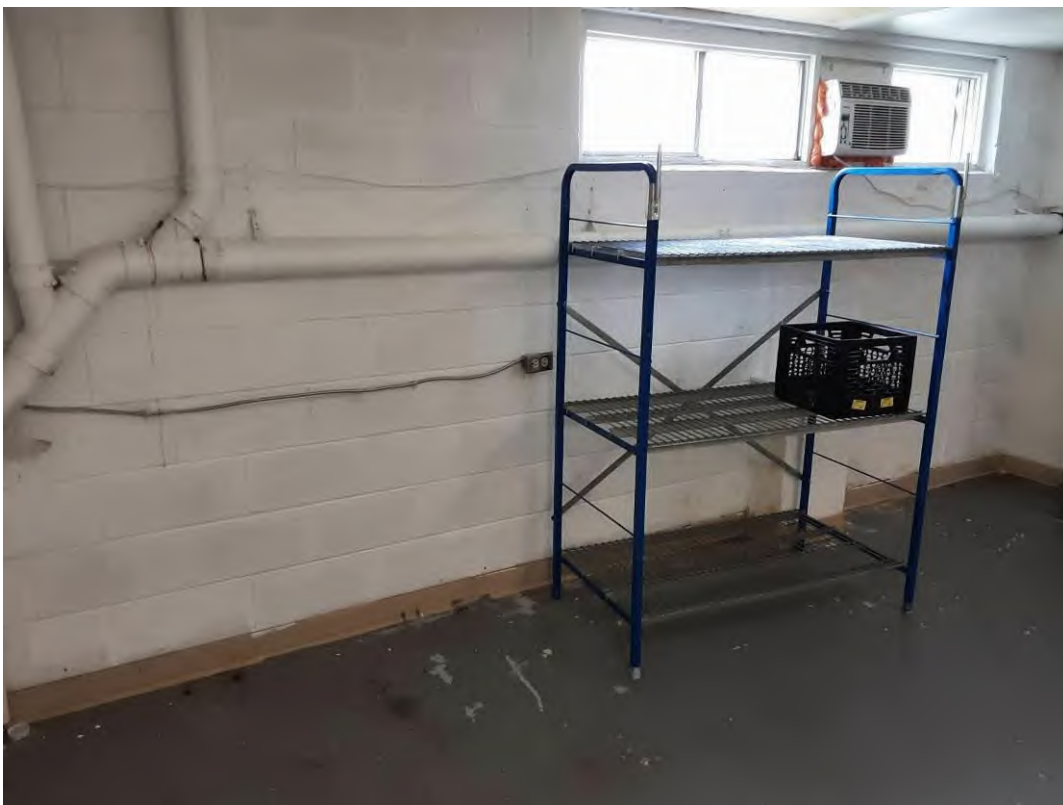
V9000 (Confirmed Asbestos), Piping, Rain Water Leader, Cement Product, Dietary Storage (Location #: 130)
