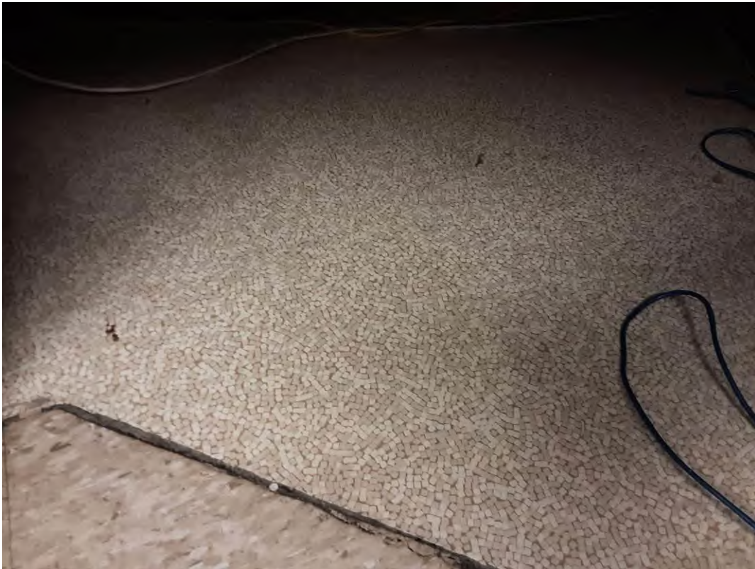
S0004A (Confirmed Asbestos), Floor, Vinyl Sheet Flooring, Lobby (Location #: 4)
