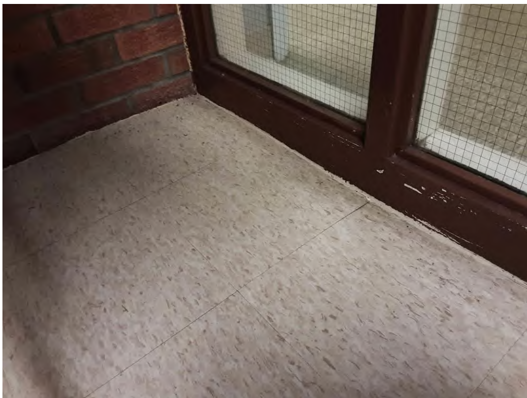
S0006A (None), Wall, Base, Caulking, Lobby (Location #: 4)
