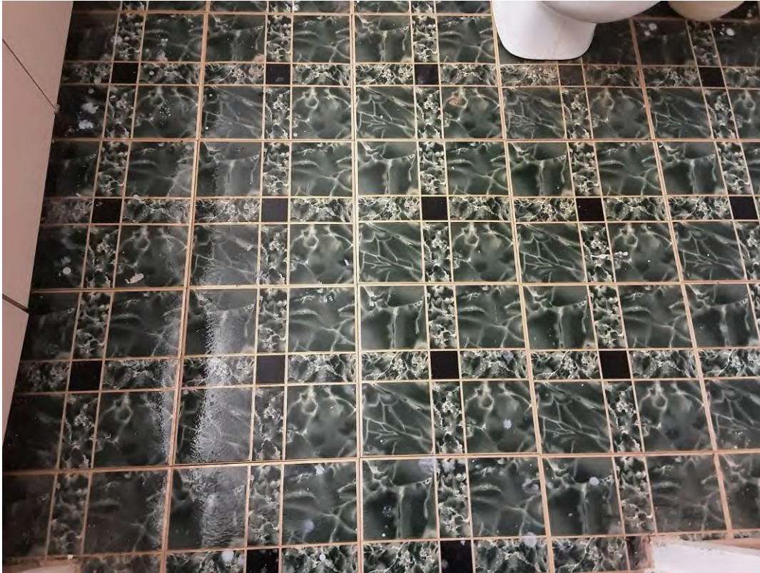
S0055C (Confirmed Asbestos), Floor, Vinyl Floor Tile and Mastic, Maintenance Supplies (Location #: 176)
