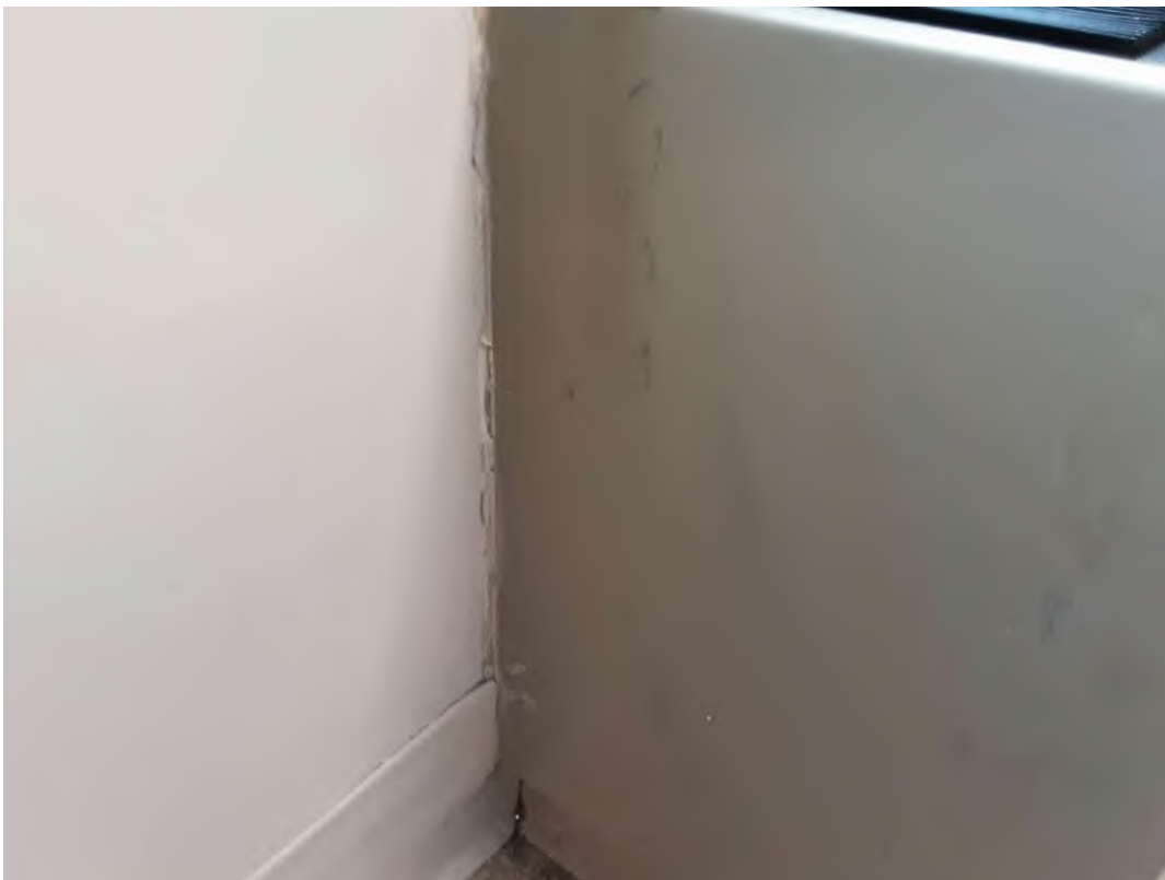
S0011A (None), Other, Radiator, Caulking, Meeting Room (Location #: 7)
