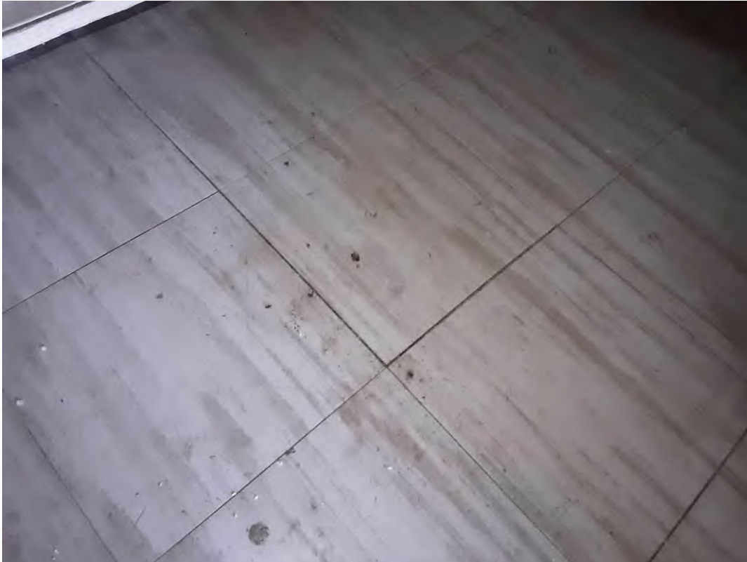
S0043A (Confirmed Asbestos), Floor, Vinyl Floor Tile and Mastic, Chemical Storage (Location #: 137)
