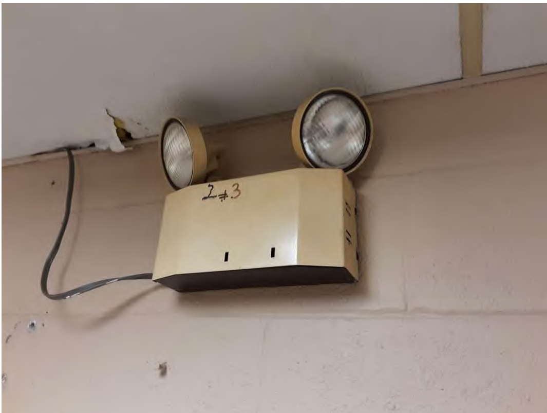
Pb Products, West Corridor (Location #: 56)
