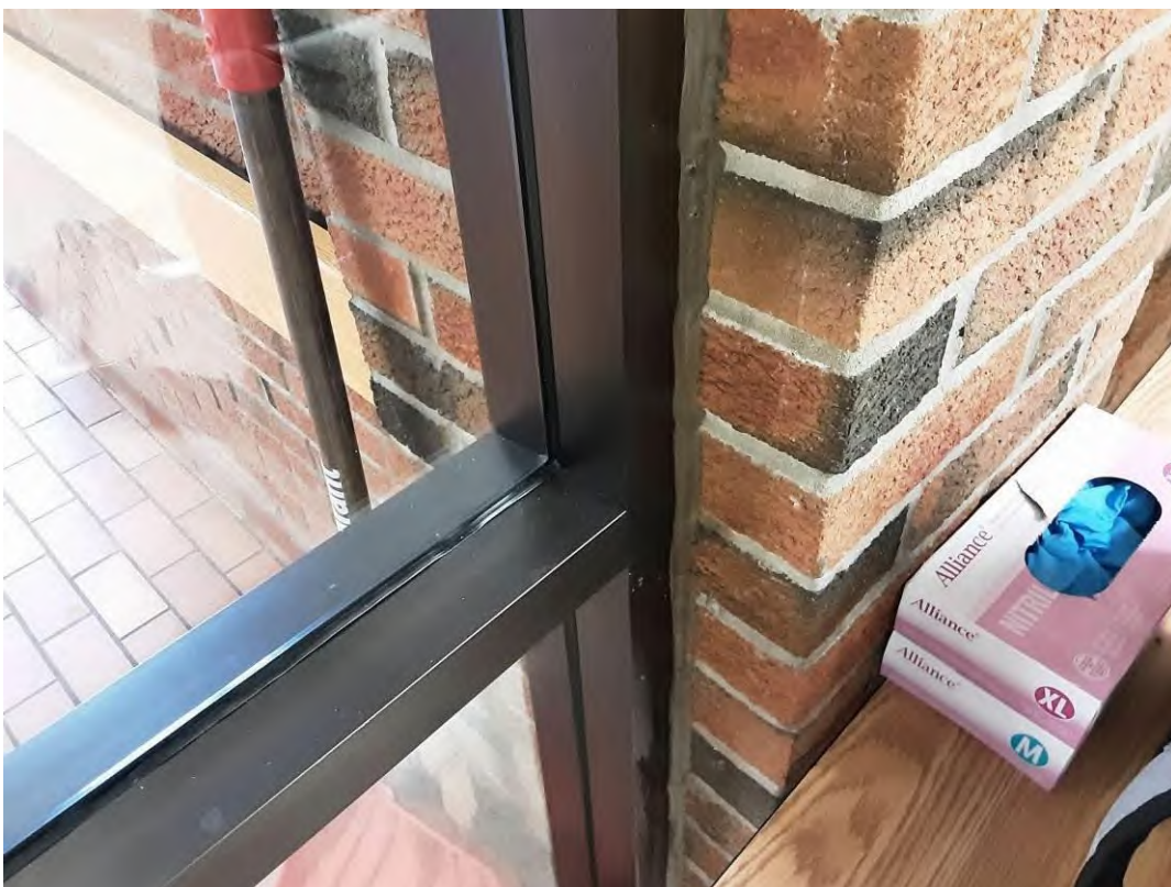
S0005A (None), Other, Door, Caulking, Lobby (Location #: 4)
