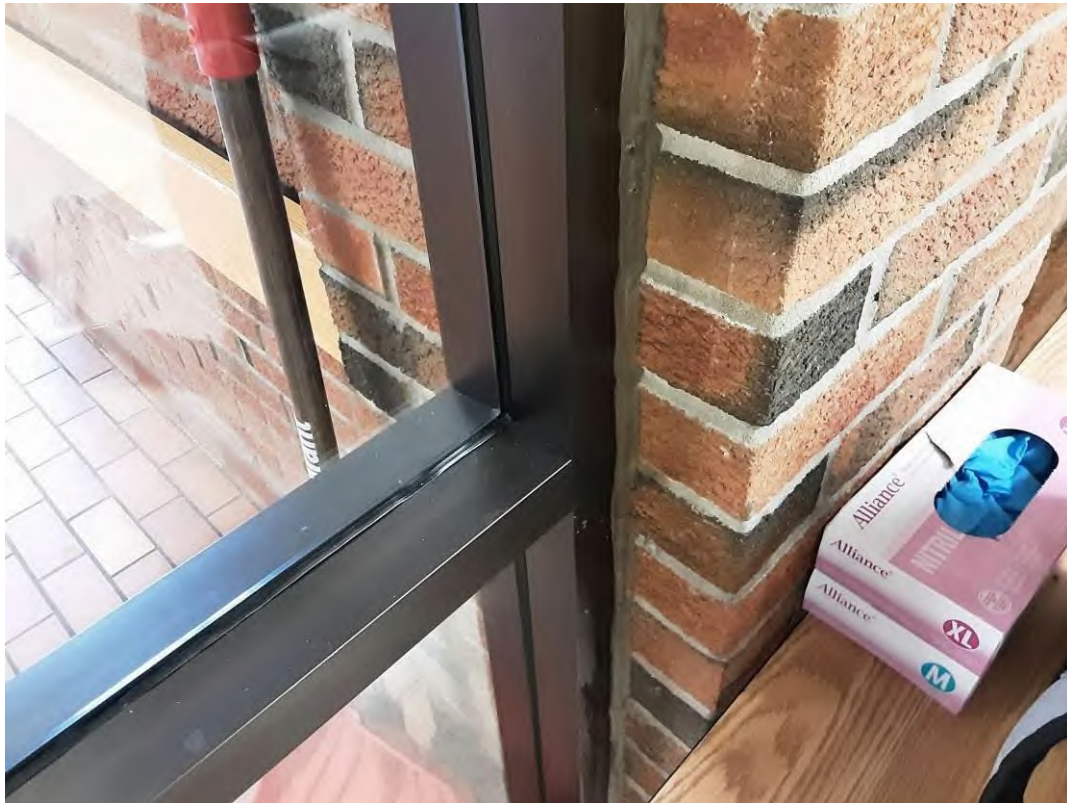
S0005A (None), Other, Door, Caulking, Lobby (Location #: 4)
