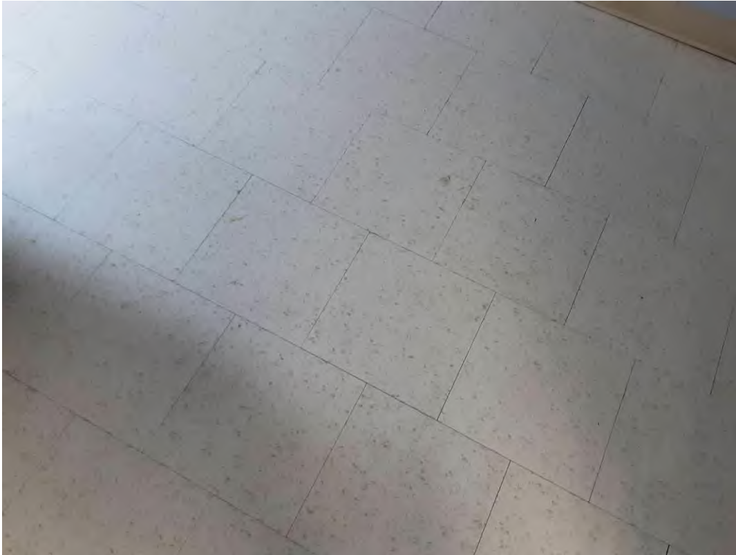
S0020A (None), Floor, All, Vinyl Floor Tile and Mastic, Tenant Room (Location #: 19)
