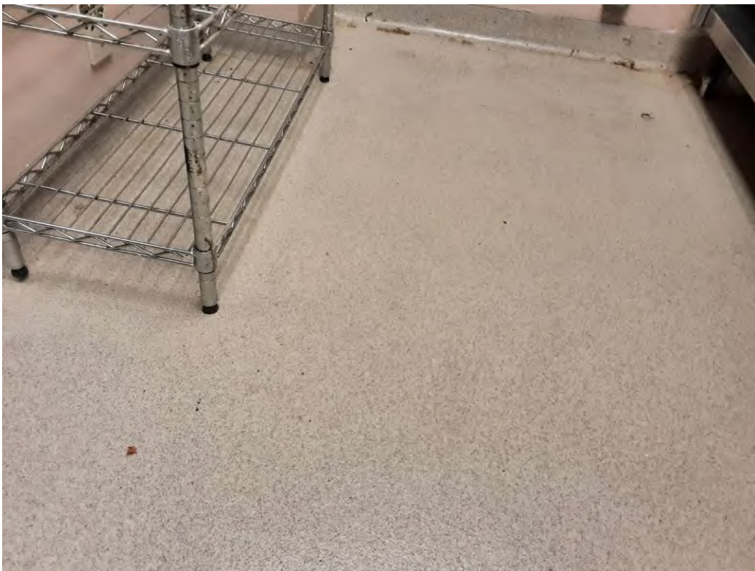
S0045A (None), Floor, All, Vinyl Sheet Flooring, Kitchen Refrigeration (Location #: 139) Resilient flooring
