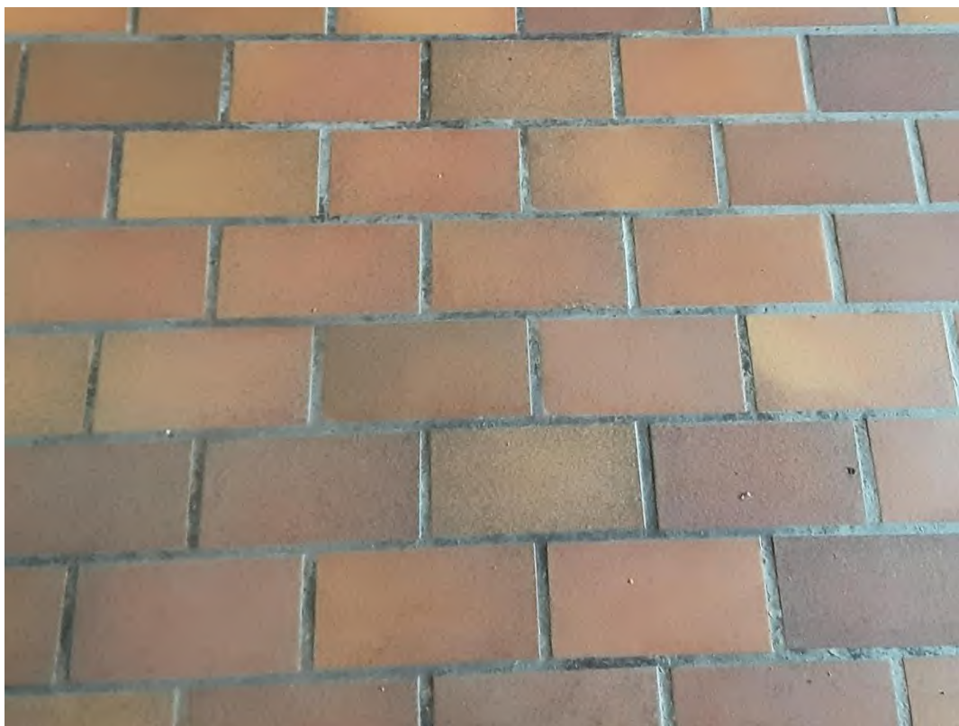
S0079A (Confirmed Asbestos), Floor, Mortar, under 2" x 6" red faux brick ceramic tile, Vestibule (Location #: 116)
