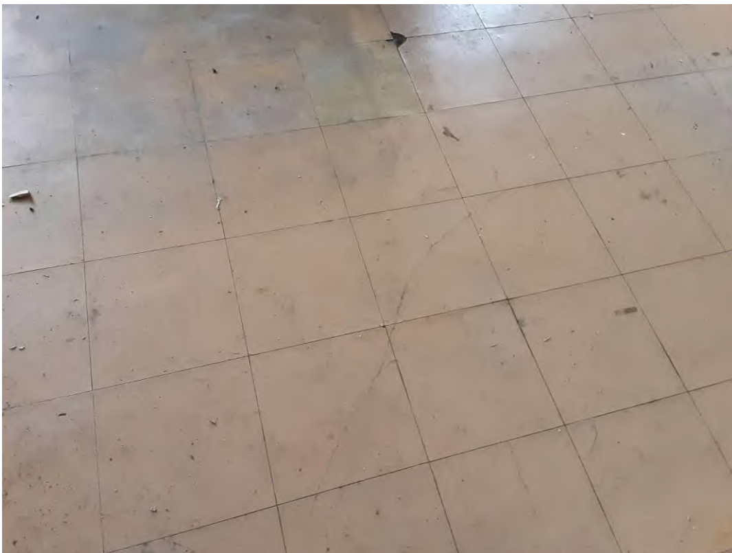
S0066C (Confirmed Asbestos), Floor, Vinyl Floor Tile and Mastic, Old House - 2nd Floor (Location #: 178)
