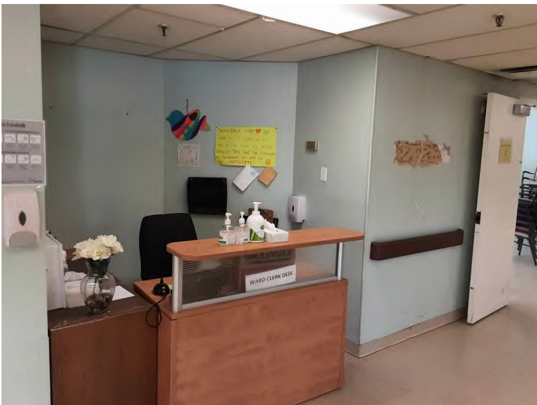
V0009 (Confirmed Asbestos), Wall, All, Drywall and joint compound, Lobby (Location #: 4)
