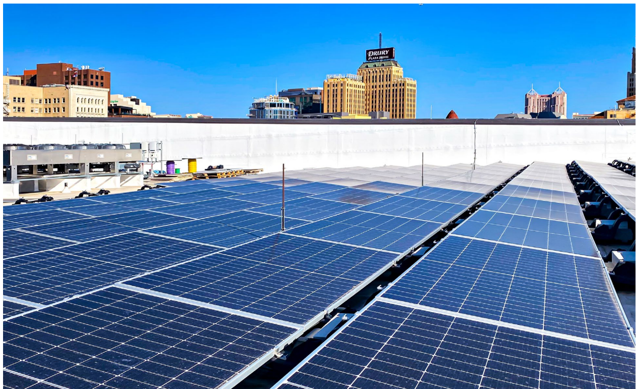
Example rooftop solar PV installation
