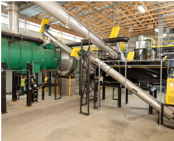
Pyrolysis Process Installed at the Morrisville Municipal Authority Facility, PA, USA (credit: Ecoremedy)
