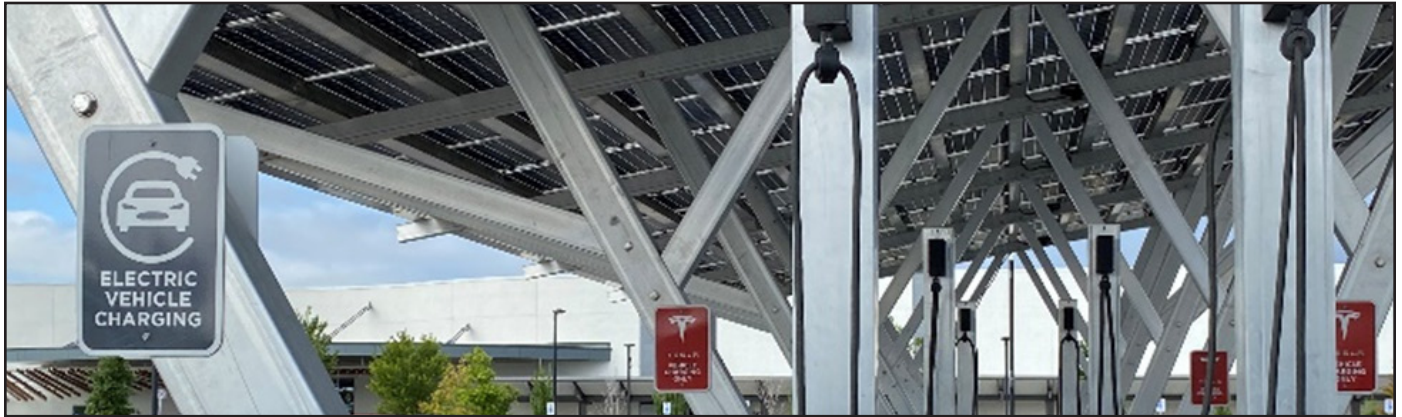
Solar panel parking structure for EV charging station
