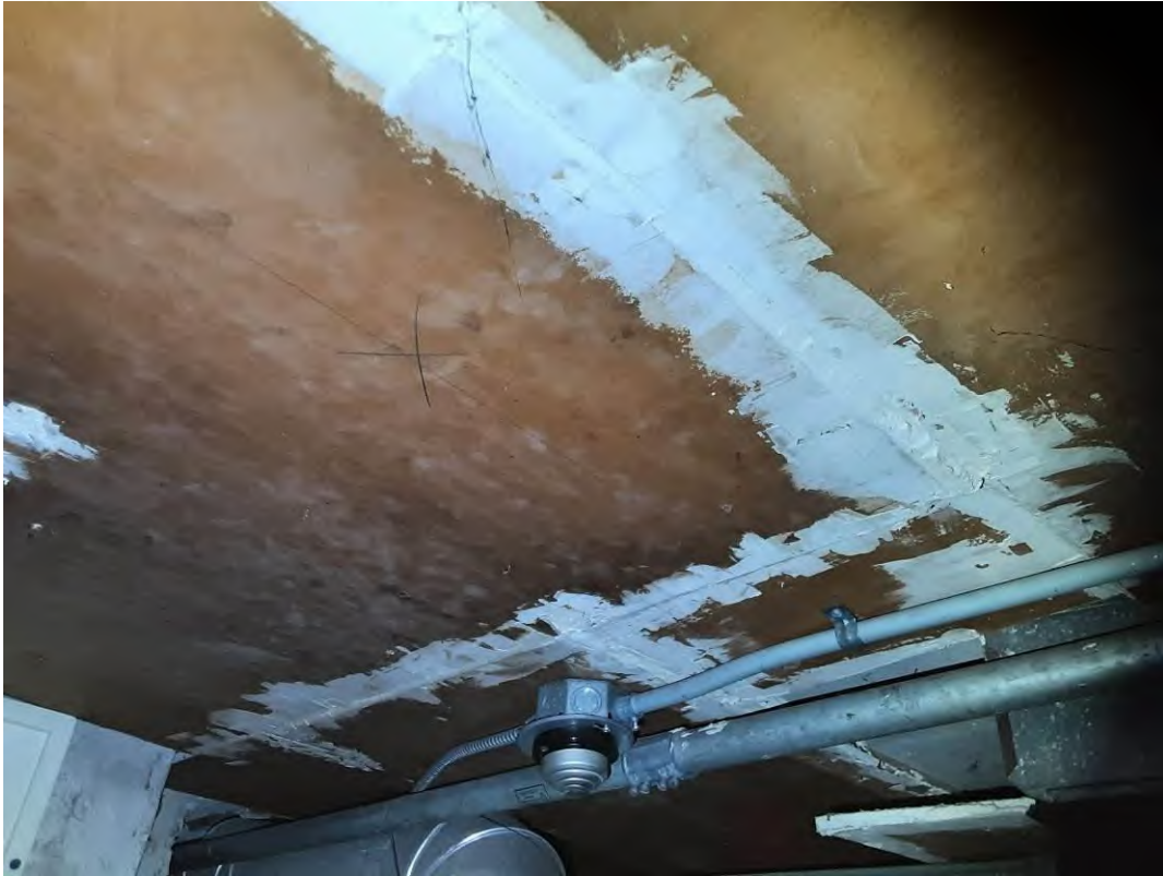
S0040A (Confirmed Asbestos), Ceiling, All, Drywall and joint compound, Old House - Basement (Location #: 135)
