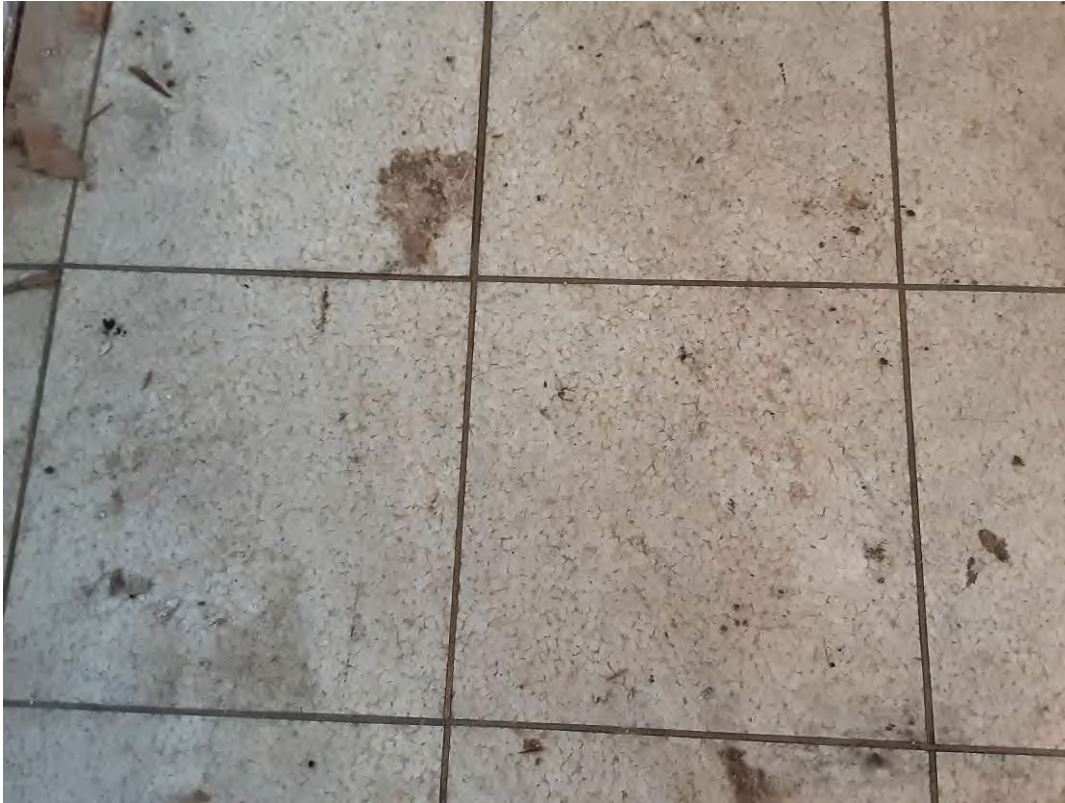
S0065C (None), Floor, Vinyl Floor Tile and Mastic, Old House - 2nd Floor (Location #: 178)
