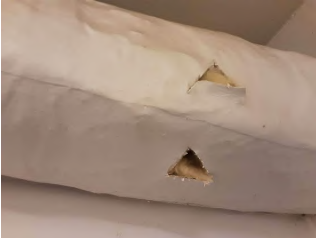
Duct, Fibreglass, Maintenance Shop (Location #: 166)
