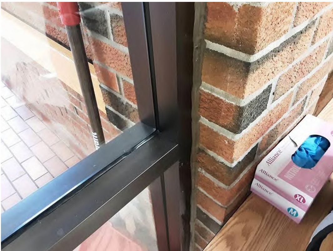
S0005A (None), Other, Door, Caulking, Lobby (Location #: 4)
