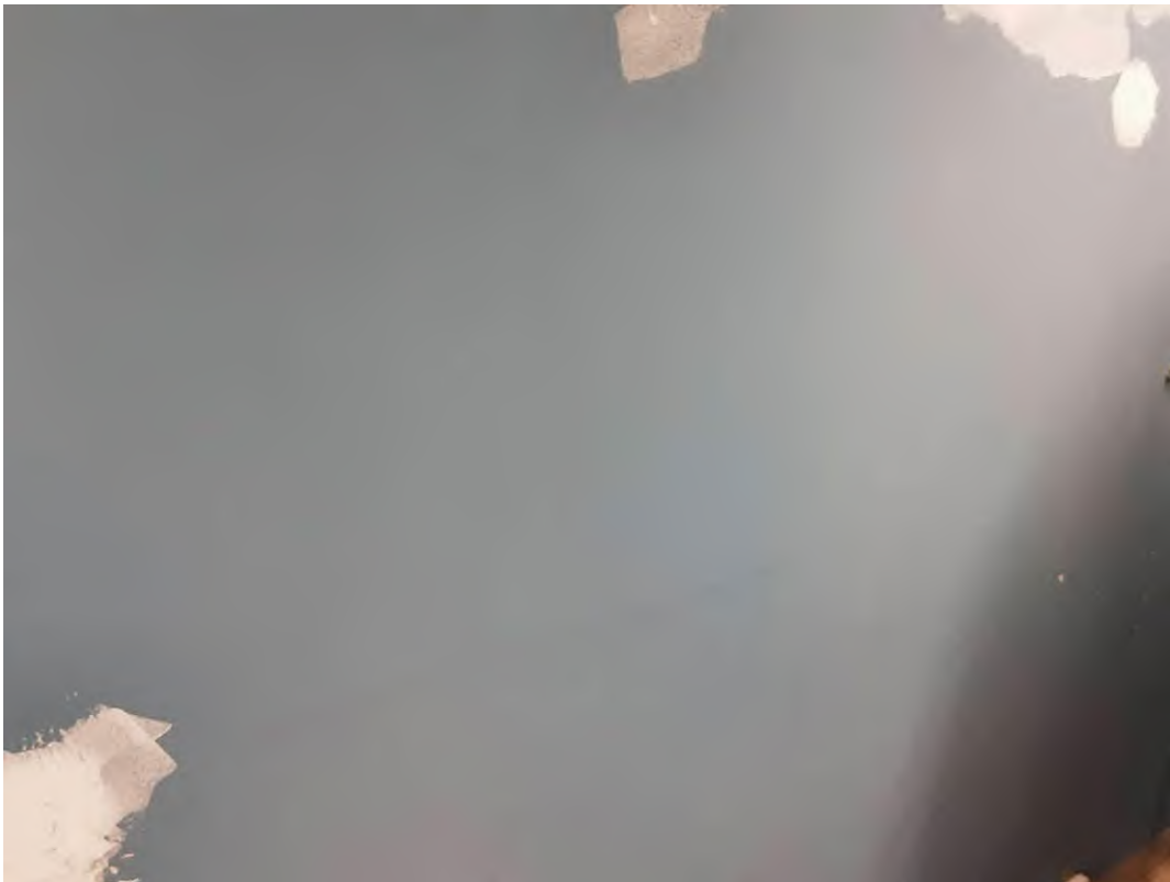
Drywall and joint compound, Blue paint on drywall, L0007, Linen Room (Location #: 27)
