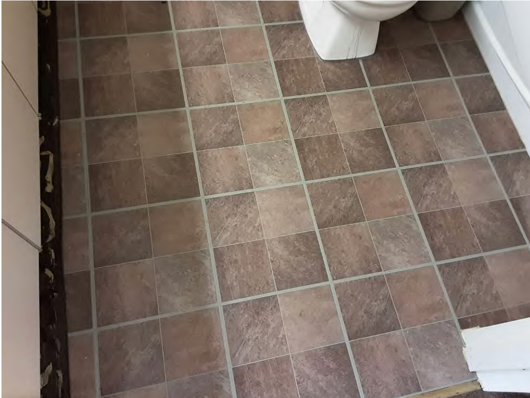
S0071C (Confirmed Asbestos), Floor, Vinyl Floor Tile and Mastic, Accounting Storage (Location #: 157)
