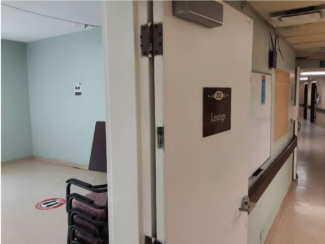
V9500 (Presumed Asbestos), Other, Door, Unidentified Material, Lounge (Location #: 11)
