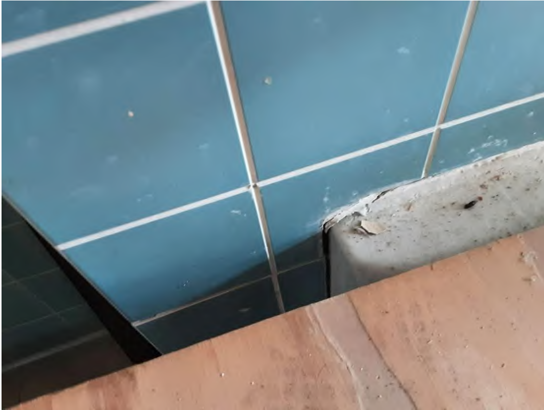
S0069C (None), Other, Caulking, Old House - 2nd Floor (Location #: 178)
