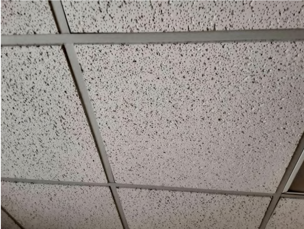
V0000 (None), Ceiling, All, Ceiling Tiles (lay-in), Meeting And Training Room (Location #: 150) Date code 1996
