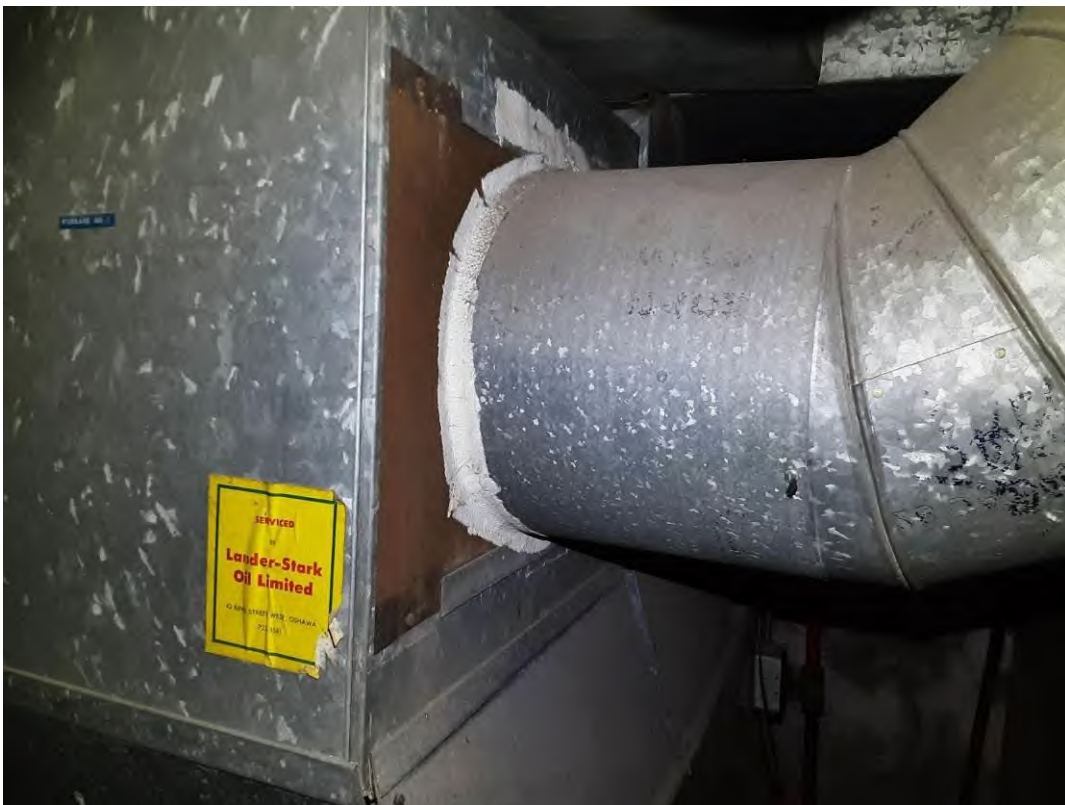
S0042A (Confirmed Asbestos), Duct, Textile, Old House - Basement (Location #: 135)
