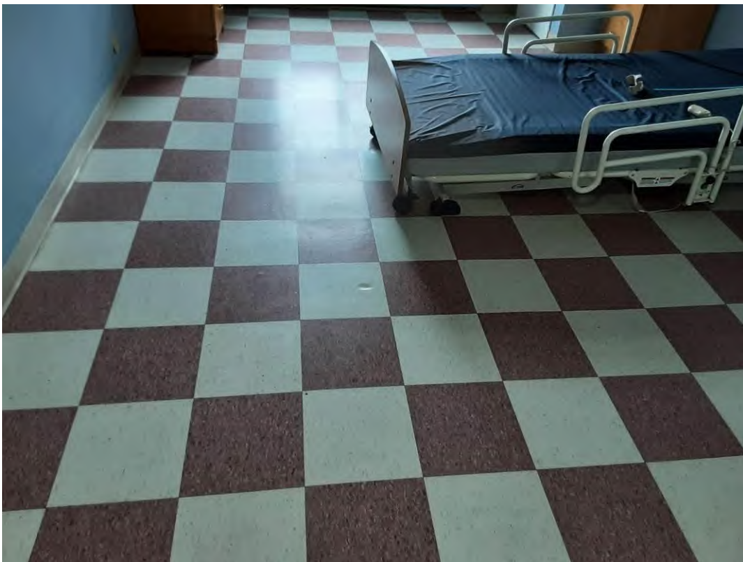
V0020 (None), Floor, All, Vinyl Floor Tile and Mastic, Tenant Room (Location #: 21)
