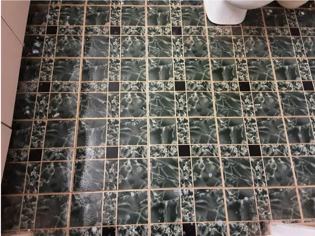
S0055C (Confirmed Asbestos), Floor, Vinyl Floor Tile and Mastic, Maintenance Supplies (Location #: 176)
