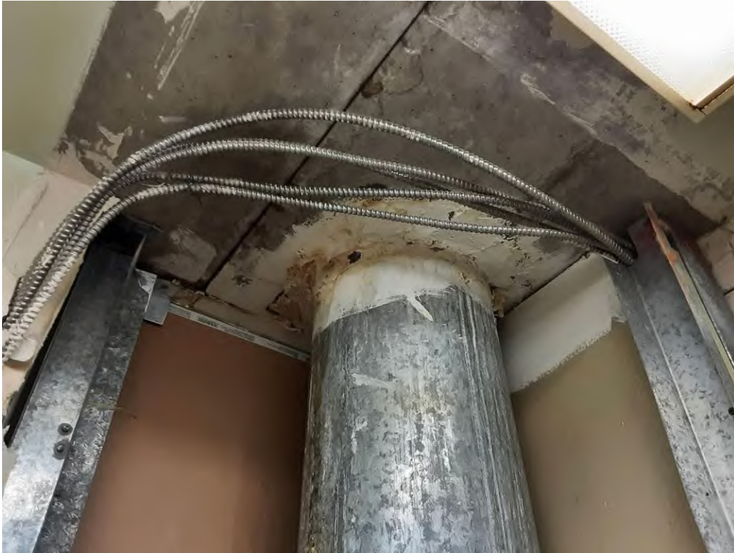
S0035A (None), Duct, Parging Cement, Utility Room (Location #: 79)
