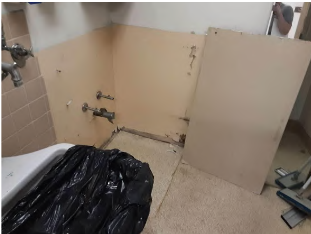
Soiled Utility Room (Location #: 152)
