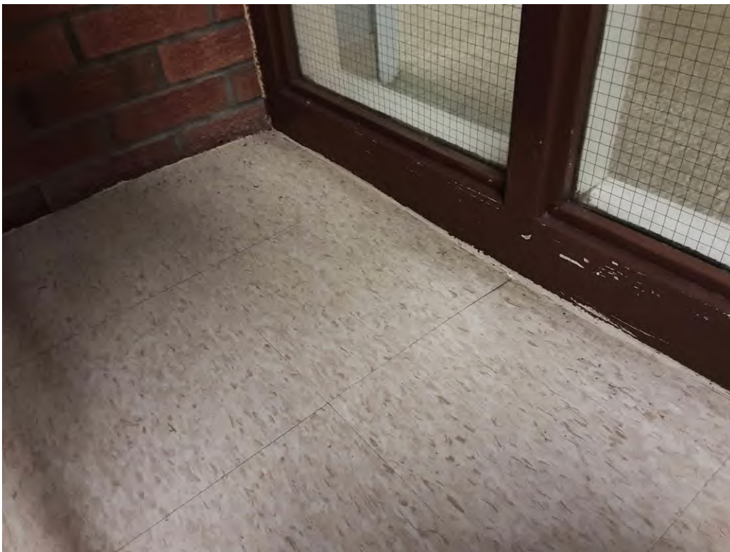
S0006A (None), Wall, Base, Caulking, Lobby (Location #: 4)
