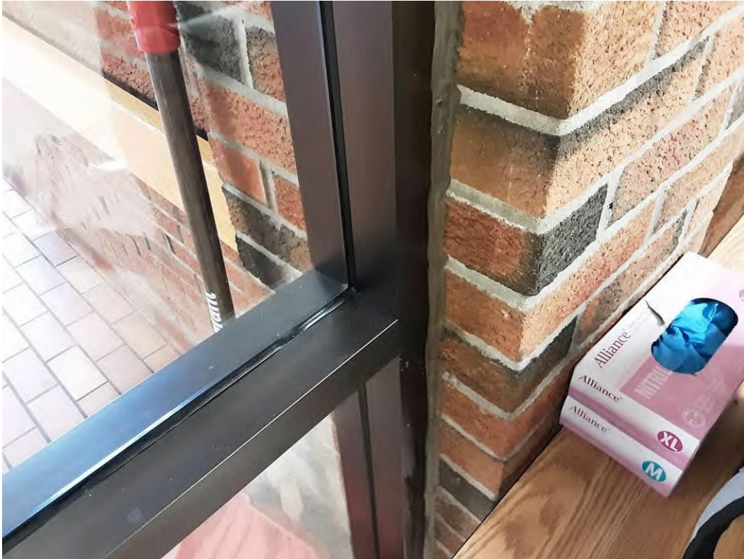
S0005A (None), Other, Door, Caulking, Lobby (Location #: 4)
