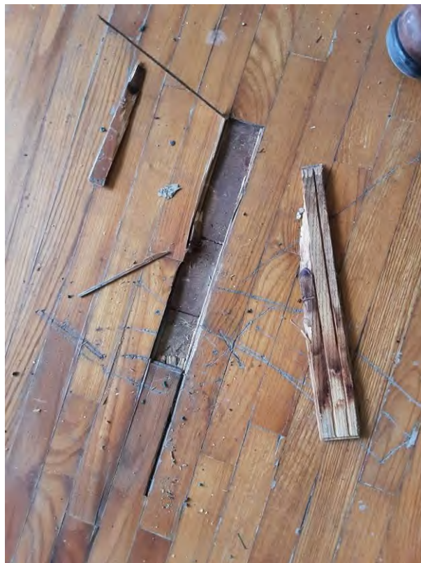
V0000 (None), Floor, Wood, Old House - 2nd Floor (Location #: 178)
