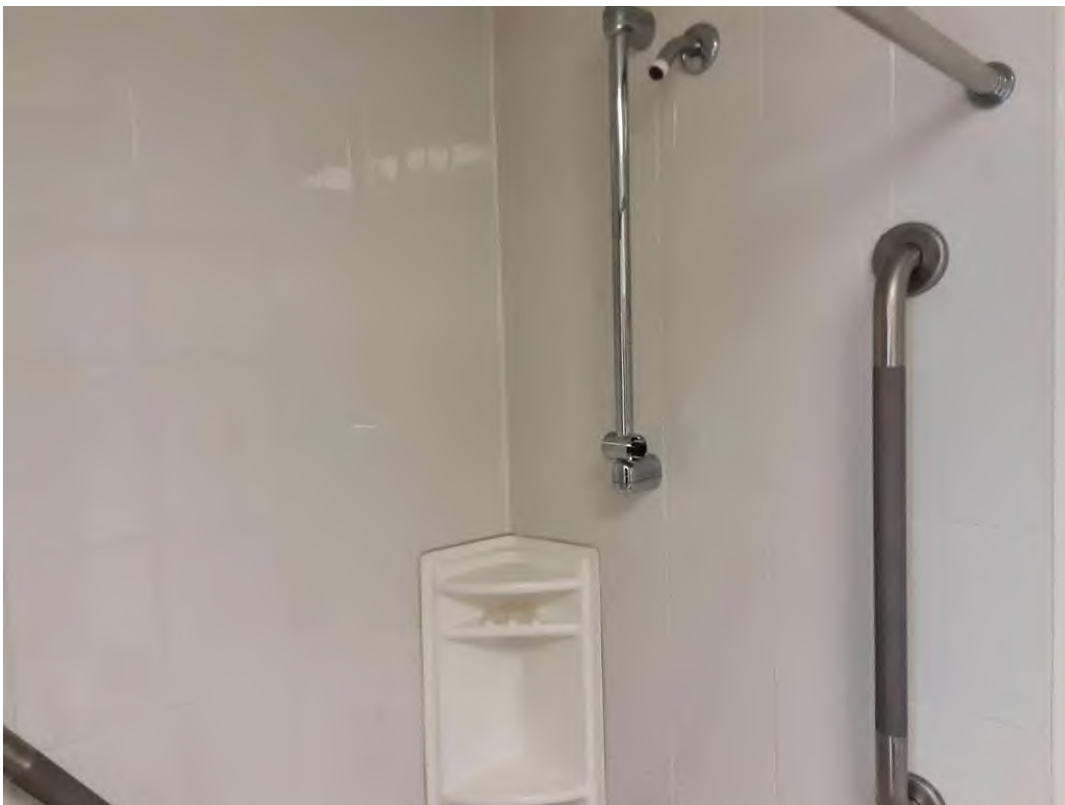
V9500 (Presumed Asbestos), Wall, Mortar, Meeting And Training Room (Location #: 150)
