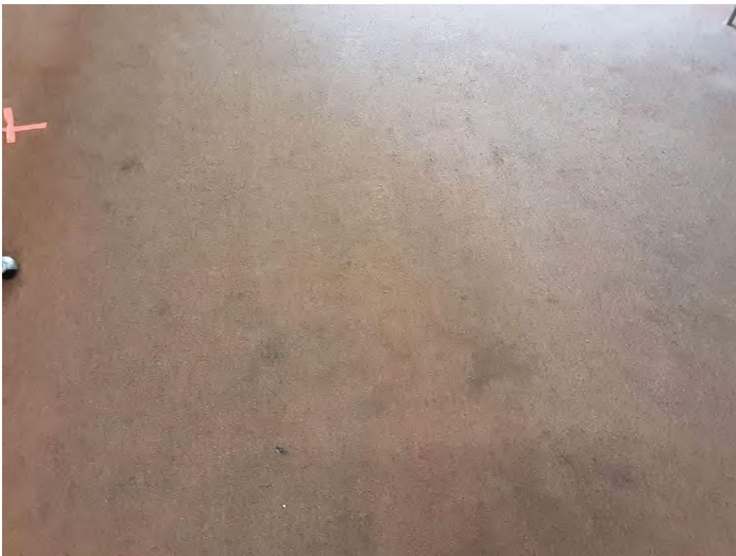
S0039A (None), Floor, Adhesive/mastic, Storage (Location #: 118)
