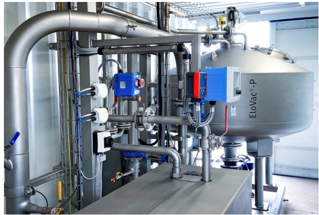
ELOVAC® Vacuum CH 4 Extraction Unit Installed at the Ejby Mølle Water Resource Recovery Facility, Odense, Denmark (credit: VCS)
