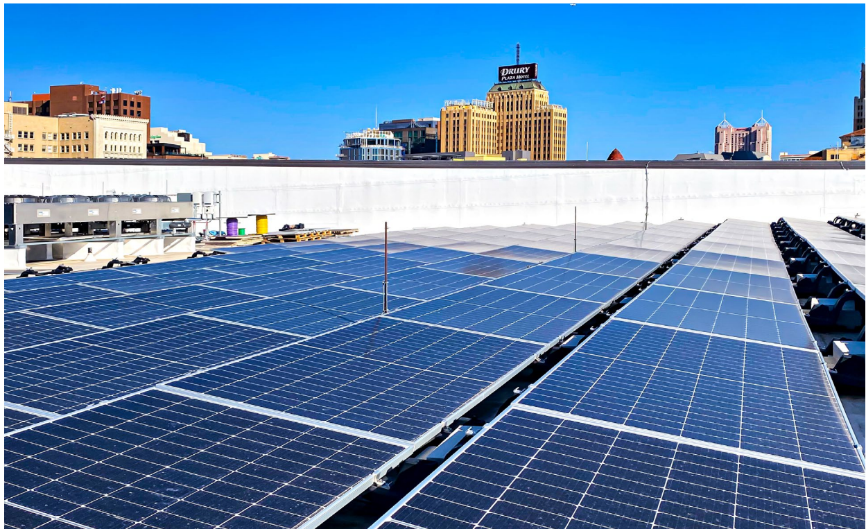
Example rooftop solar PV installation
