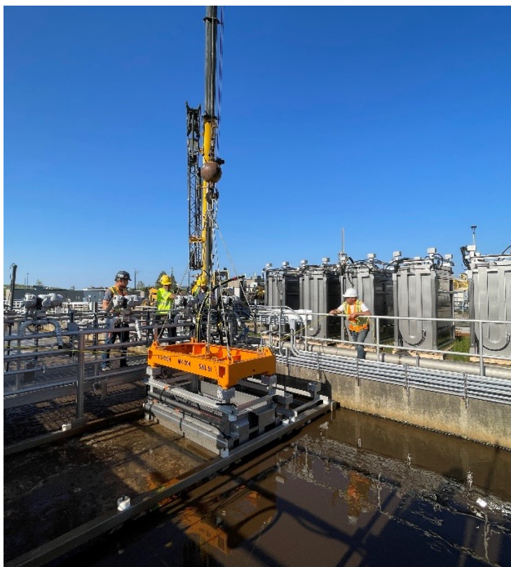
Installation of MABR Modules at the Elmira Wastewater Treatment Plant, Region of Waterloo
